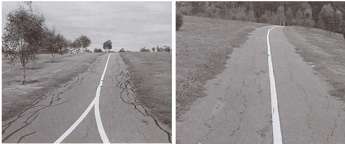
Figure F 1: Asphalt paths requiring maintenance
